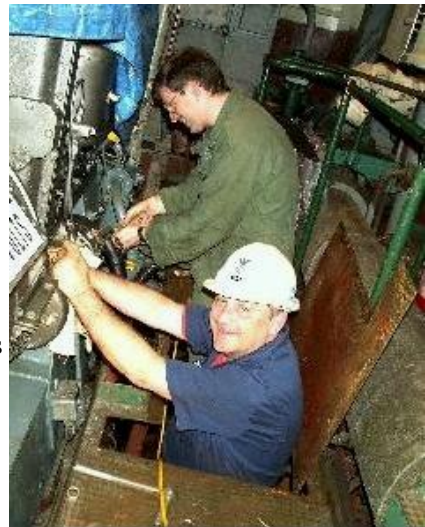
Gus Negus and Barry Witte prepare the emergency diesel.
