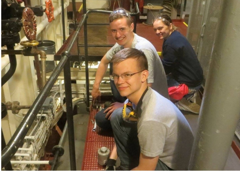
RPI Midshipmen John Obermiller, Nathan Arntz, and Isabel Donelson worked replacing missing handrails in the aft motor room.
