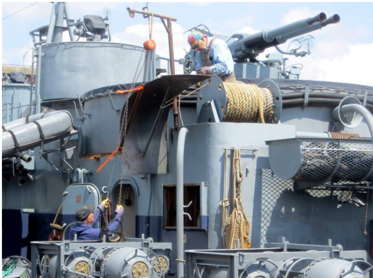
Doug and the shipfitters began fitting in the first section of the aft supply fan vent intake.
