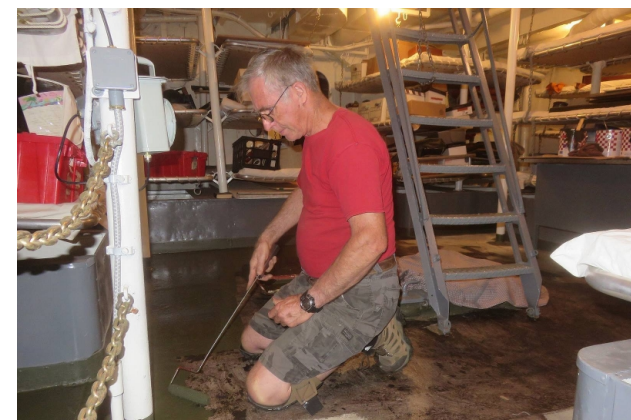
Gary Sheedy and Thomas Scian painted out the deck in compartment C-203-L.
