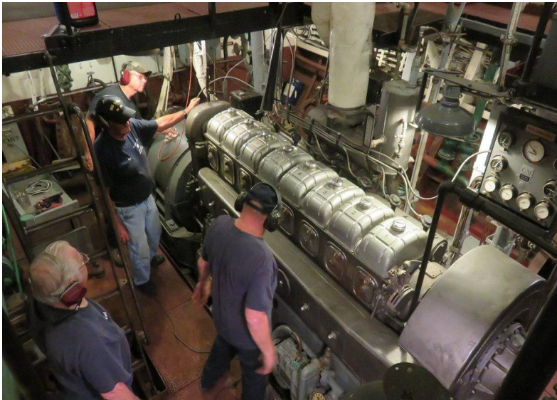
B-3 Genset test run.
