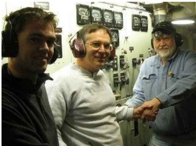
Brian Goodman, Barry Witte and George Gollas monitor the power generation of the aft distribution board.
