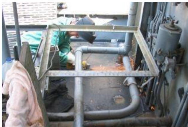
On the flying bridge Tim Benner is hard at work patching holes in the deck.
