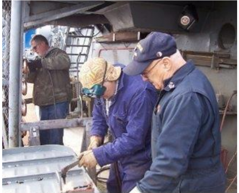
Dave Jeffries works cleaning the reefer deck coils as Doug Tanner and Dave Mardon repair a watertight door.
