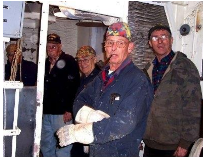
Haggart, Mardon, Benner and Sheedy making sure Doug gets the scullery sink back in level.
