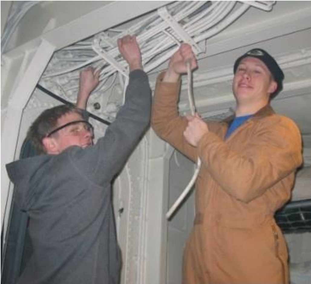
Jack Lyons and James Conlon work to run new armored cable for the forward ventilation.
