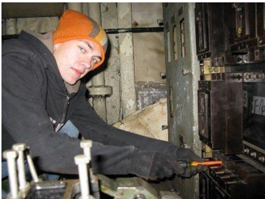
Brian Goodman, EE student at WPI , installing a circuit breaker in the forward switchboard to better serve power directly to a welding machine. The breaker Brian is installing is one of the ones he retrieved from LSM-45 in May 2009. The LSM lives on in the form of parts on Slater.
