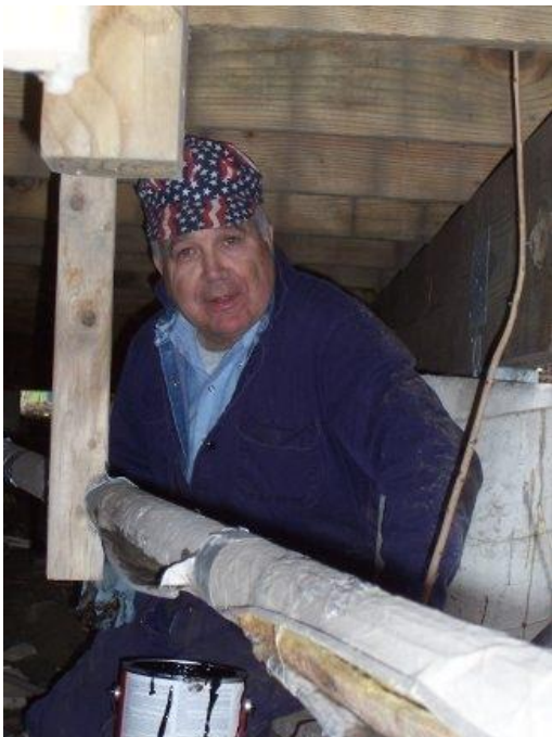
Doug "Don't forget me" Tanner insulating water lines under the observation deck.
