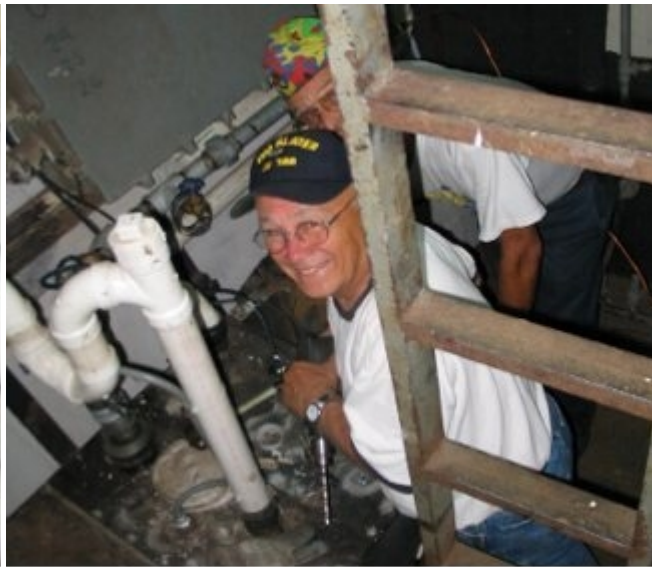
Super Dave Mardon and Tim Benner put the finishing touches on the forward septic tank.
