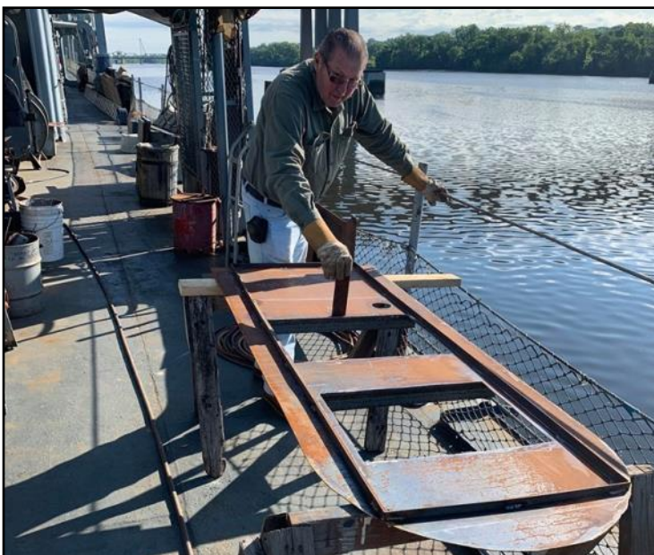
Danny fabricated a new door for Officer's Country to fit air conditioners.
