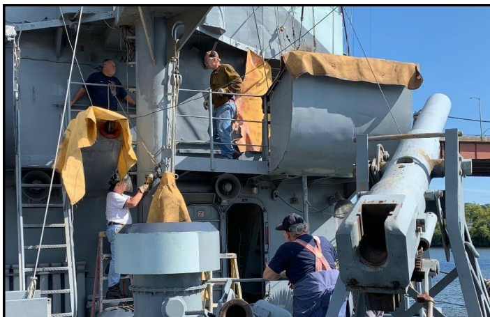
It takes a lot of welding blanket to move a bell. Chuck and Dave Wasson got the new bracket welded and primed.
