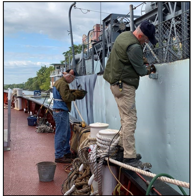
Using the HARVEY as a work float Dave and Chuck did some welding and grinding.
