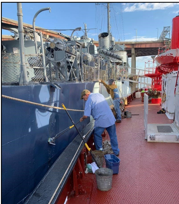
Walt and Warren scrubbed the rust streaks off of the hull from the HARVEY.
