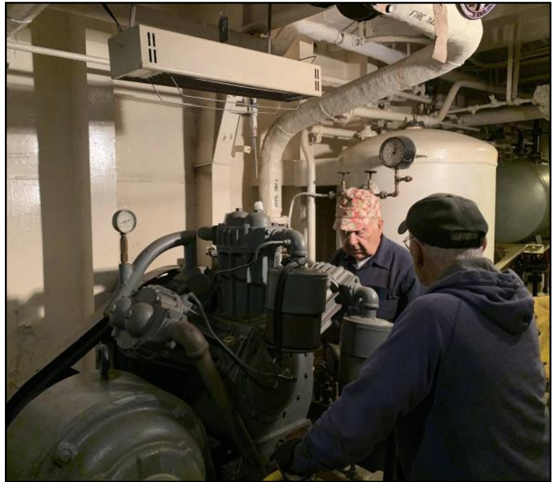
Our main air compressor is out of action. Doug and Super Dave are working to get it repaired so we can use the air tools.
