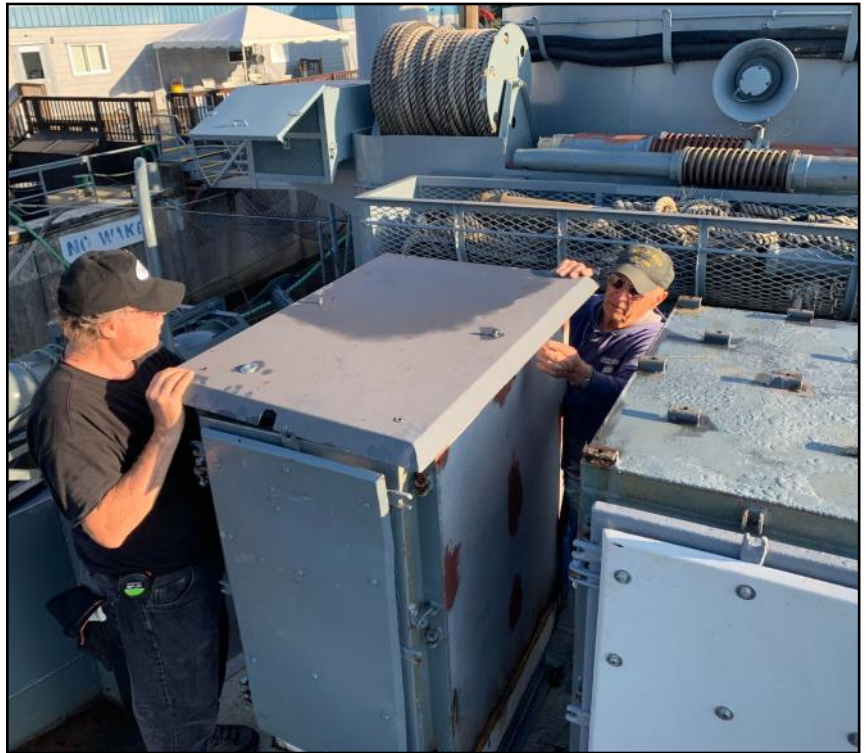
The shipfitters mounted the heat shields on the gun 33 ready service lockers.
