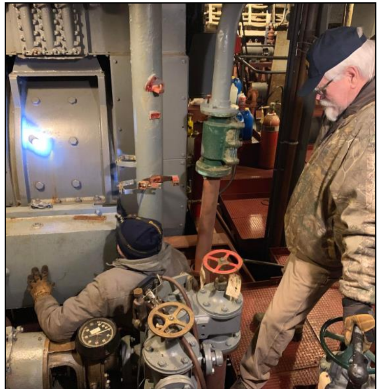
There is no break here. It's just as cold in the engine room as it is outside.
