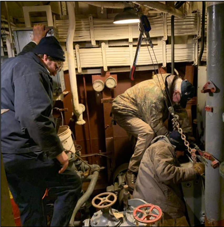
Our engineering gang removed the fire pump priming tank to access the area under the generators.
