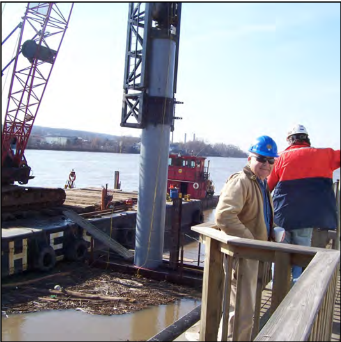
Doug Tanner and Spec Consulting supervised the installation of the mooring dolphins.
