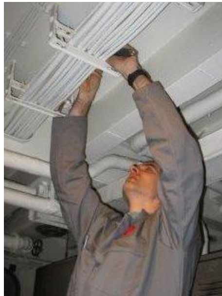
Jim Hewitt works on opening a cable-way to allow removal of old cable.
