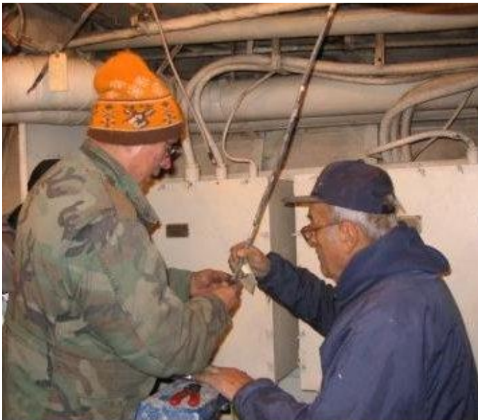
Ken Kaskoun and Bob Callender splicing in a new 1MC cable outside the CPO Mess.
