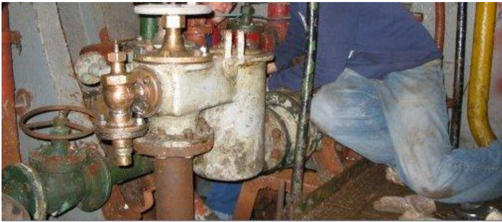
RPI NROTC students John Camp and Kevin Guldner at work in B1 repairing the bilge pump system.
