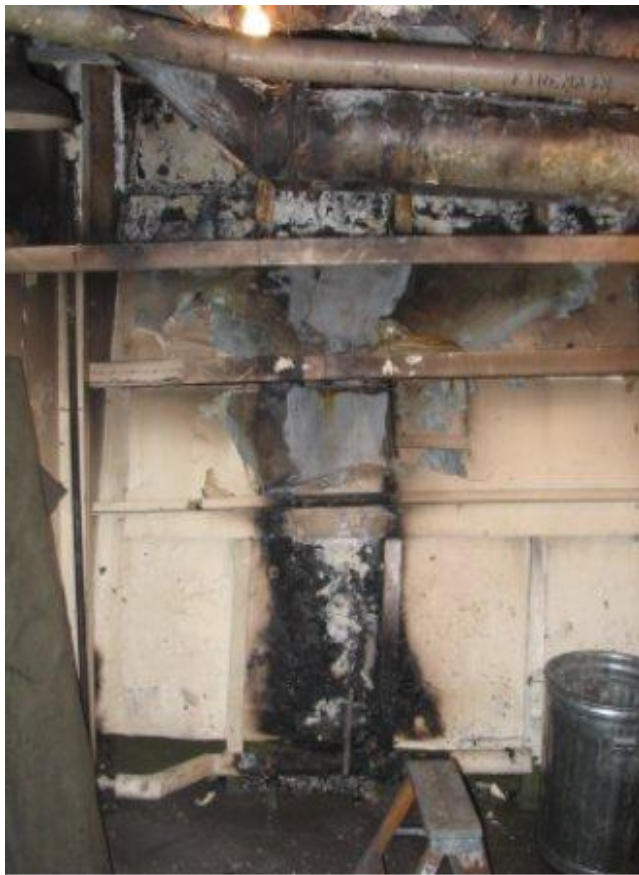
Fire damage - starboard side.
