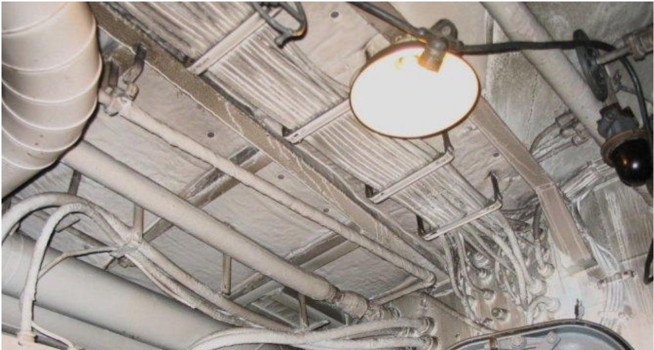
Overhead smoke damage in the forward passageway. The CPO Mess looks much the same.
