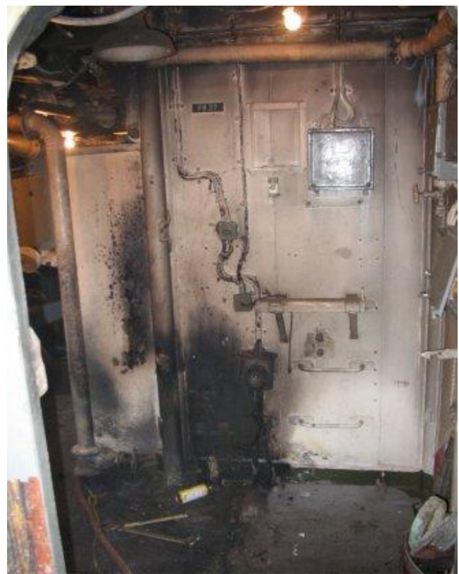
Fire damage - port side.
