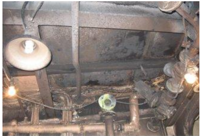
Overhead fire damage - port side.
