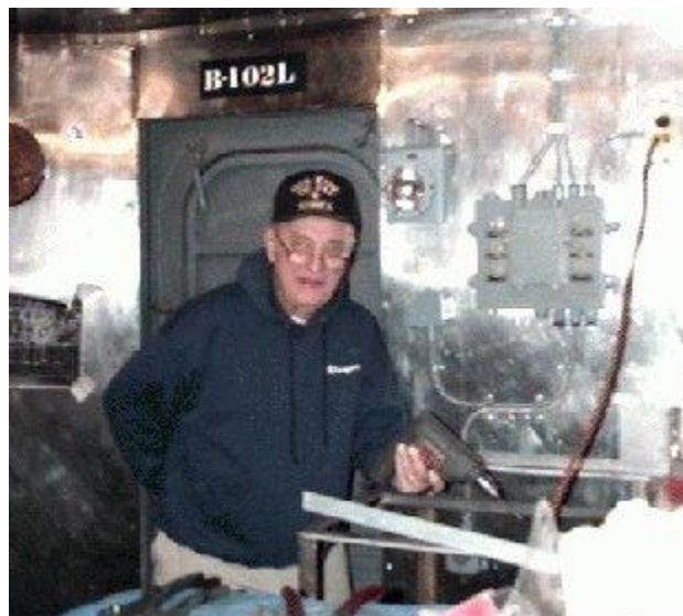
Bob Callender works on pop riveting stainless back on to the galley bulkheads.
