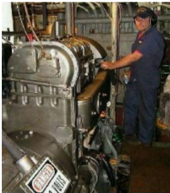
Gus Negus running the Emergency Diesel.
