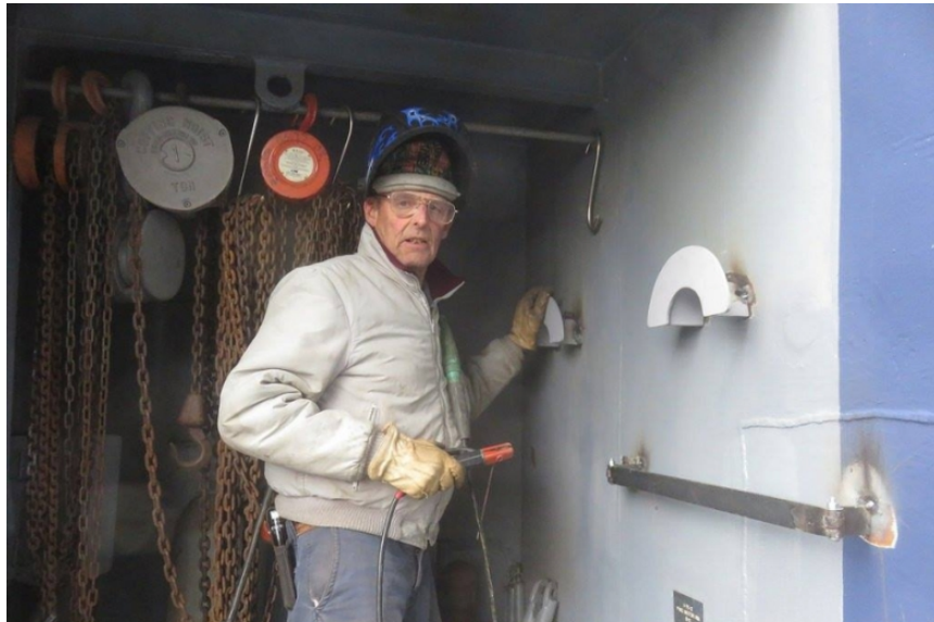
Tim Benner welding up a new hose rack to replace one that had been removed.
