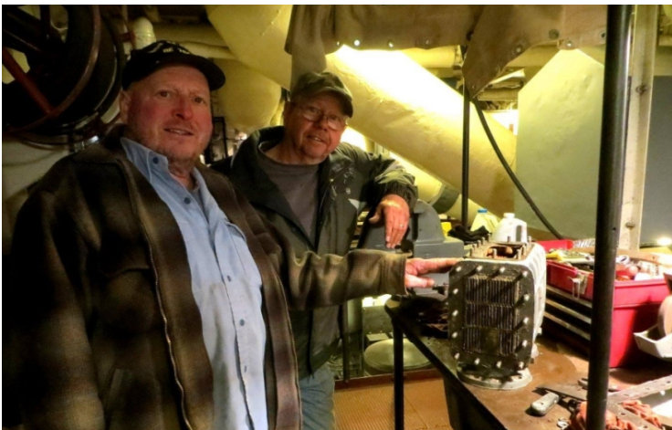
Engineers Mike and Gary ponder what to do about their heat exchanger.
