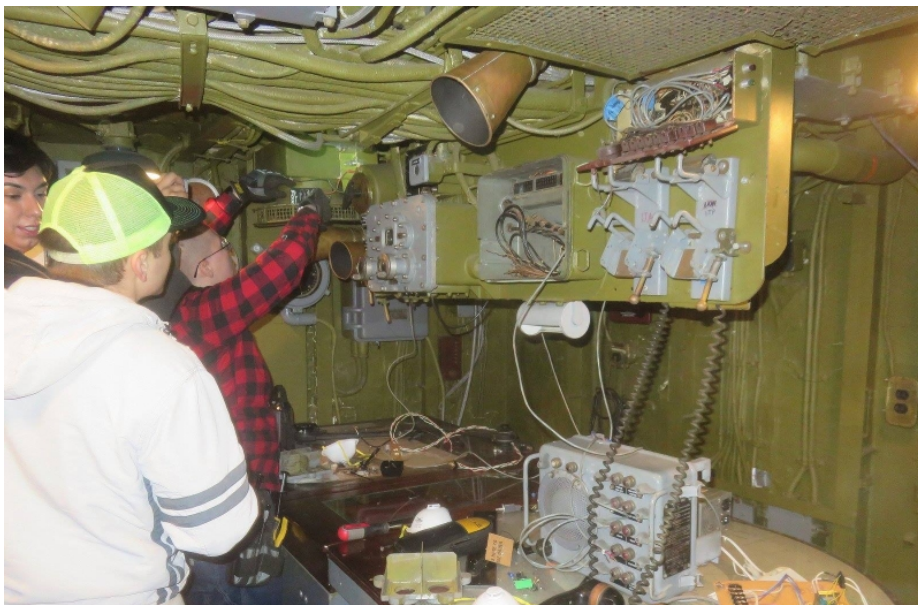
Volunteer Sailors from Ballston Spa have been rewiring CIC.
