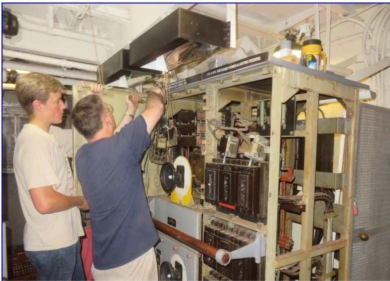
Volunteers Jim Lenden and Barry Witte overhauling the emergency diesel distribution board.
