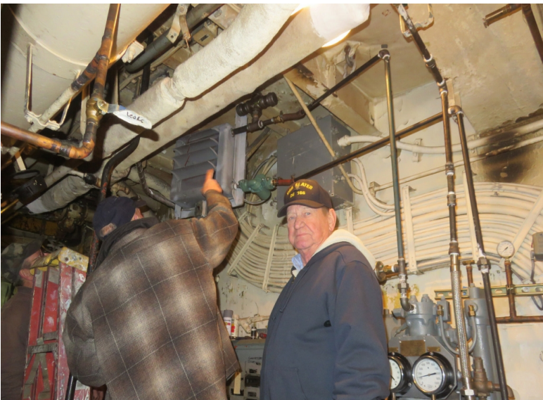
Engineers Mike Dingmon and Ken Myrick tweaking the cooling radiator on the new HP air compressor.
