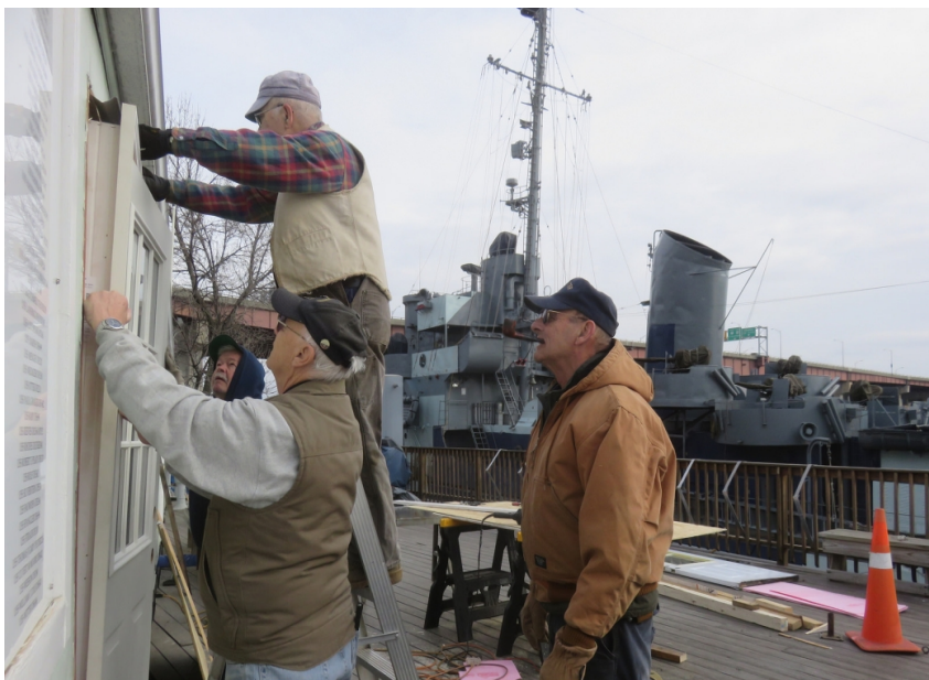
Doug Tanner's crew installing the new store door as part of the trailer renovations.
