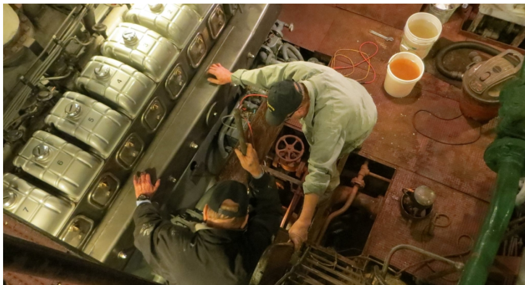
Test run of the B-3 ship's service generator.
