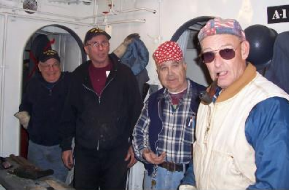
The brain trust, Mardon, Sheedy, Tanner and Benner, trying to figure out how to cut the expansion joint gasket.
