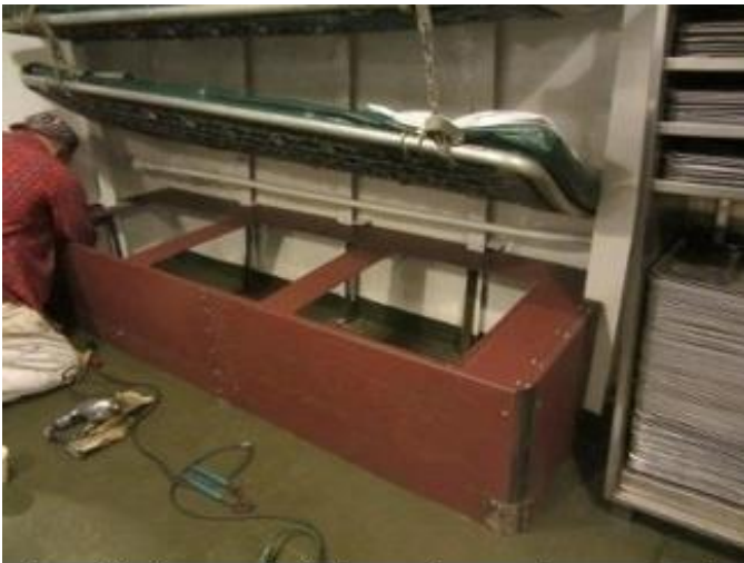
The Shipfitters fabricated a replacement for the missing bunk locker on the messdeck.
