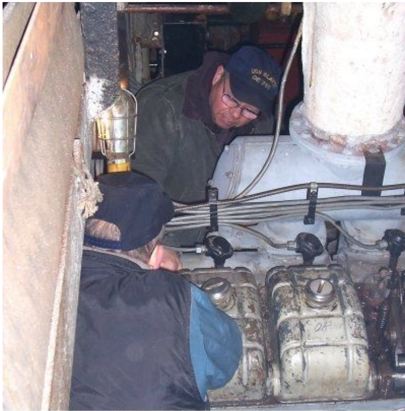
Gus Negus and Gary Lubrano continue work on the aft ship's service generator.
