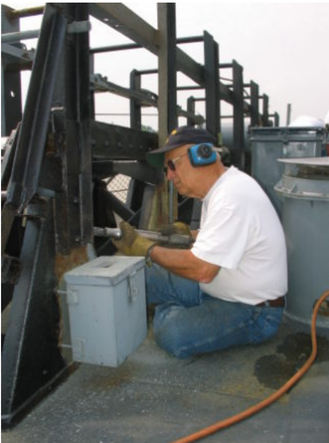
Chipping the starboard fantail rack has been a major summer project. As always, Dave was right in the middle of the action!
