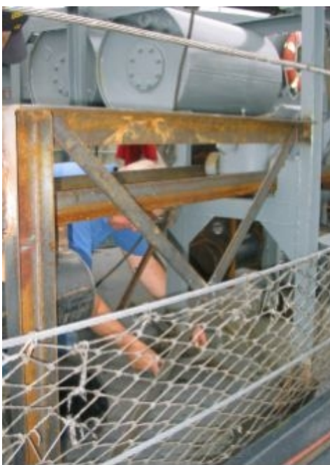
Gene Jackey, a good friend of Dave, tack welds parts on to a new K-gun rack.
