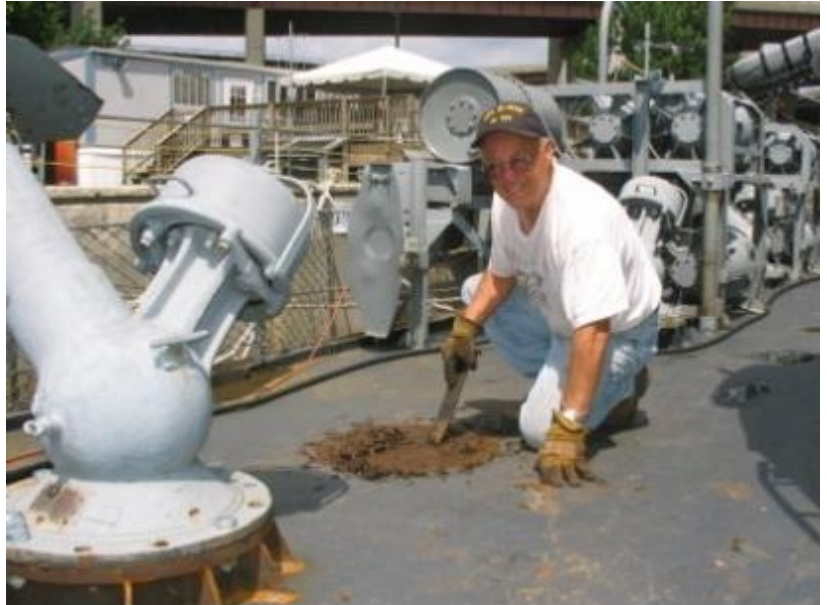
After moving a K-gun we found a large round rust spot where it had been. Dave went right at it with a chipping tool quickly getting the mess cleaned up!
