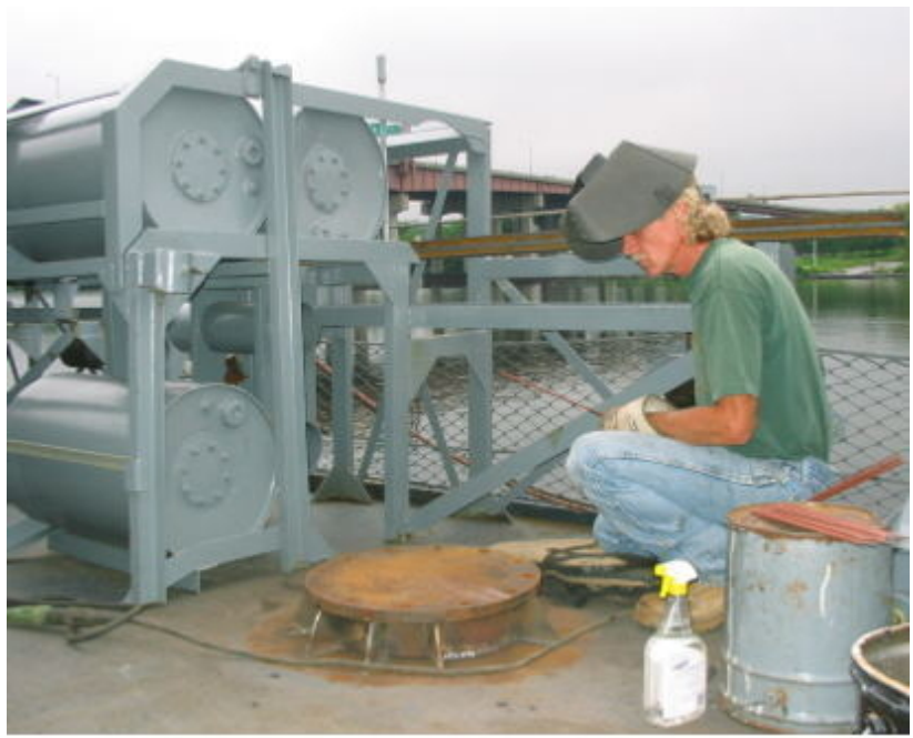
Dave stood the always vital and under appreciated firewatch as welder Bob Bareis welded K-gun racks and bases to the deck!
