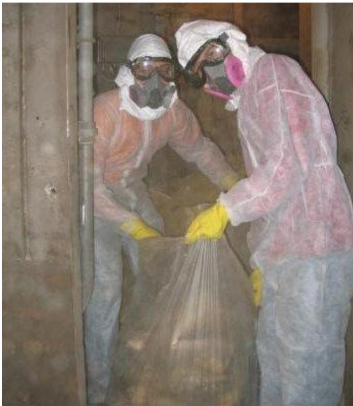
Continuing on the "masking" theme, Austin Jolly and Brian Schuessler bag the filthy remains of five month worth of work in the forward passageway.
