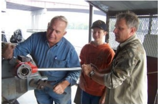
Three generations of Parkers, Jim, Zac and Joe threading pipe for the forward head.
