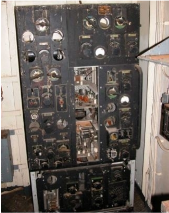
Before: The TBL radio transmitter that Tom Horsfall is restoring in California...
