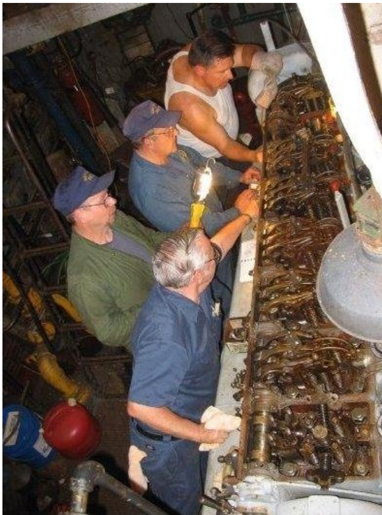
Engineers Karl Herchenroder, Gary Lubrano, Gus Negus and Bill Siebert going over the injectors on the aft ship's service generator
