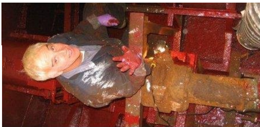
Finishing up the port shaft alley. More exciting work like this will happen during the winter.
