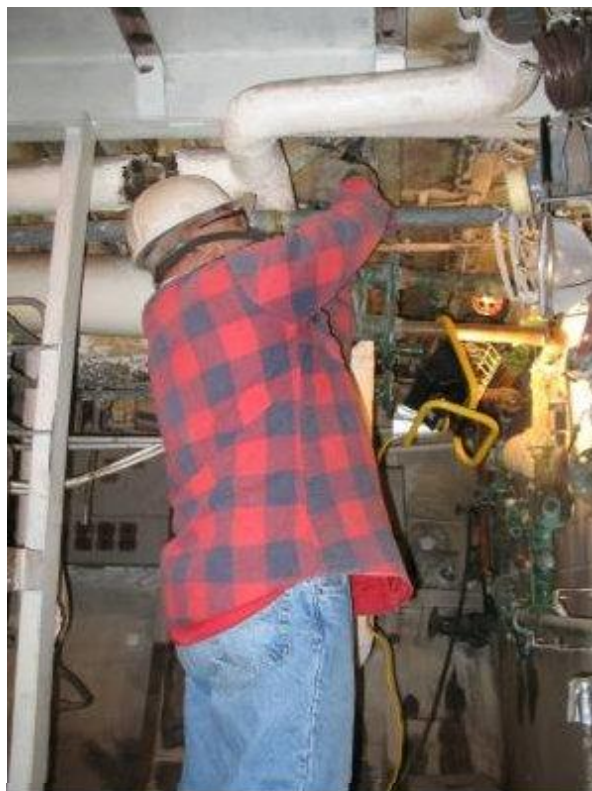
Chris Fedden keeps Gary Sheedy happy by chipping the reefer deck overhead.
