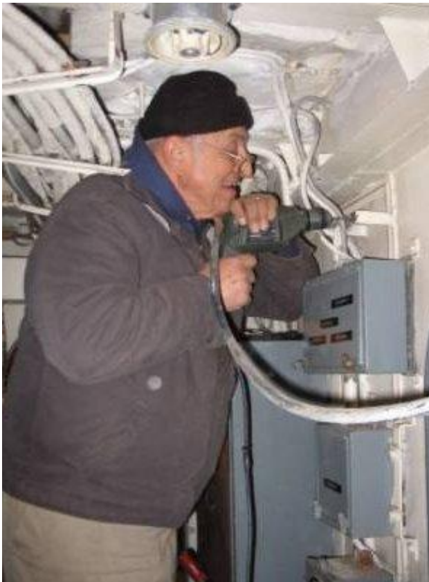
Bob Callender drills a hole for a cable clamp in the aft passageway.
