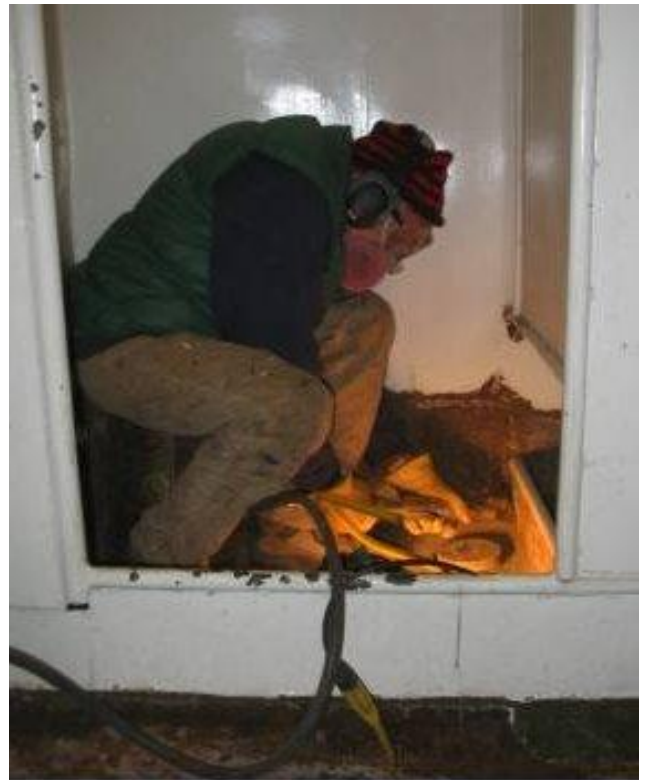
Rocky Rockwood chips the shower deck and the bottom of the bulkheads.
