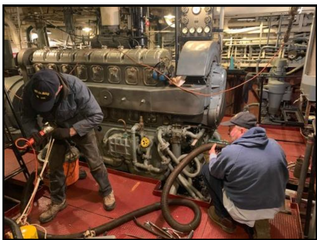
Karl, Larry and Mike winterized the diesel generators .
