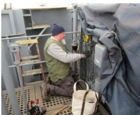
Steve Klauck pulling wires on the flying bridge prior to replacement of stuffing tubes.
