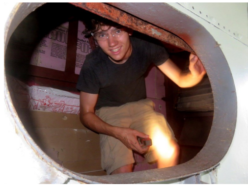
Rewiring the signal lamp, step two, on the hottest day of the year. Of course, the wires run through the fan room.
