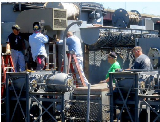
Work has been completed on the aft supply vent intake. We just need it to stop raining so we can paint it.
