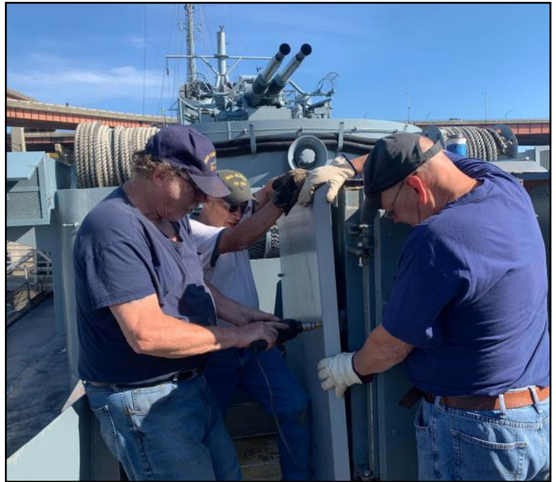
Warren, Earl, and Dale finished mounting the heat shields on the ready service lockers.
