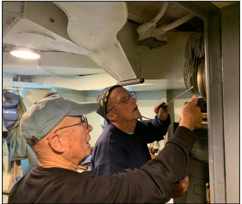
Ken and Larry work on installing a compartment fan in the Ship's Office.
