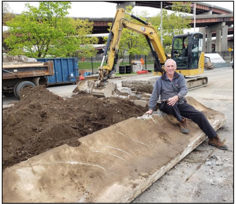
Gary sure is excited to be rid of the "island" in the parking lot.
