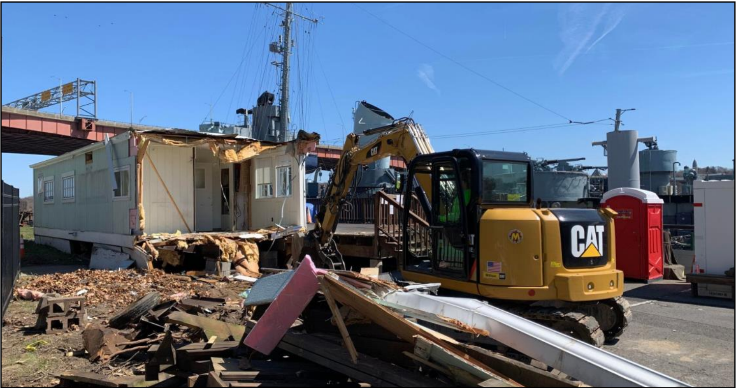
The trailer demolition was an exciting stage of the Shoreside Facilities Project.
