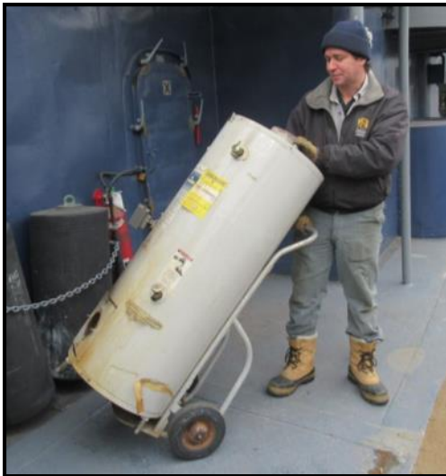
Bye bye, hot water heater. You've served us well for twenty years, but it's time to replace you.
