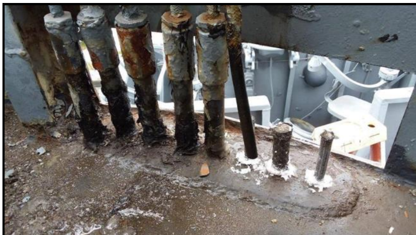
The shipfitters continued work on the wasted stuffing tubes in the gun director tub.
